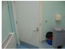
Missing grab bar
