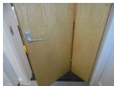
Missing grab bar
